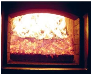
Blick in den Kessel
